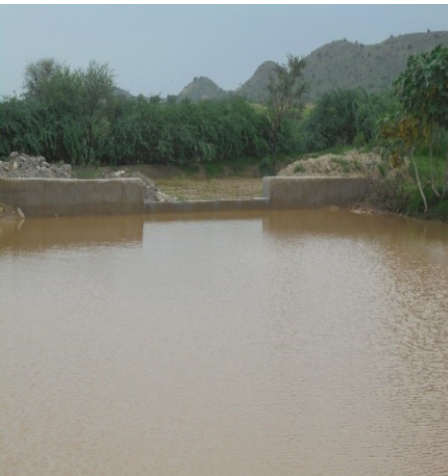
Below: Water management through waste weir
